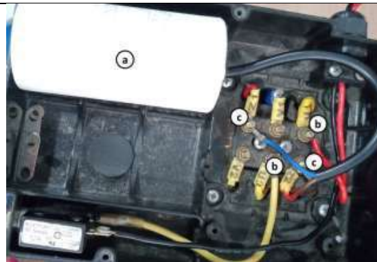
Figure. 3 Excitation Capacitor Installation (a) 40 \mu\text{F} Capacitor (b) Primary Winding Terminal (c) Auxiliary Winding Terminal
